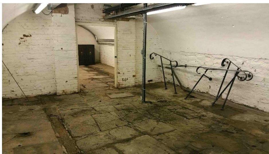
Example of large cellar rooms in Area B – note flagstone floor and multiple drainage channels (Location 20)
