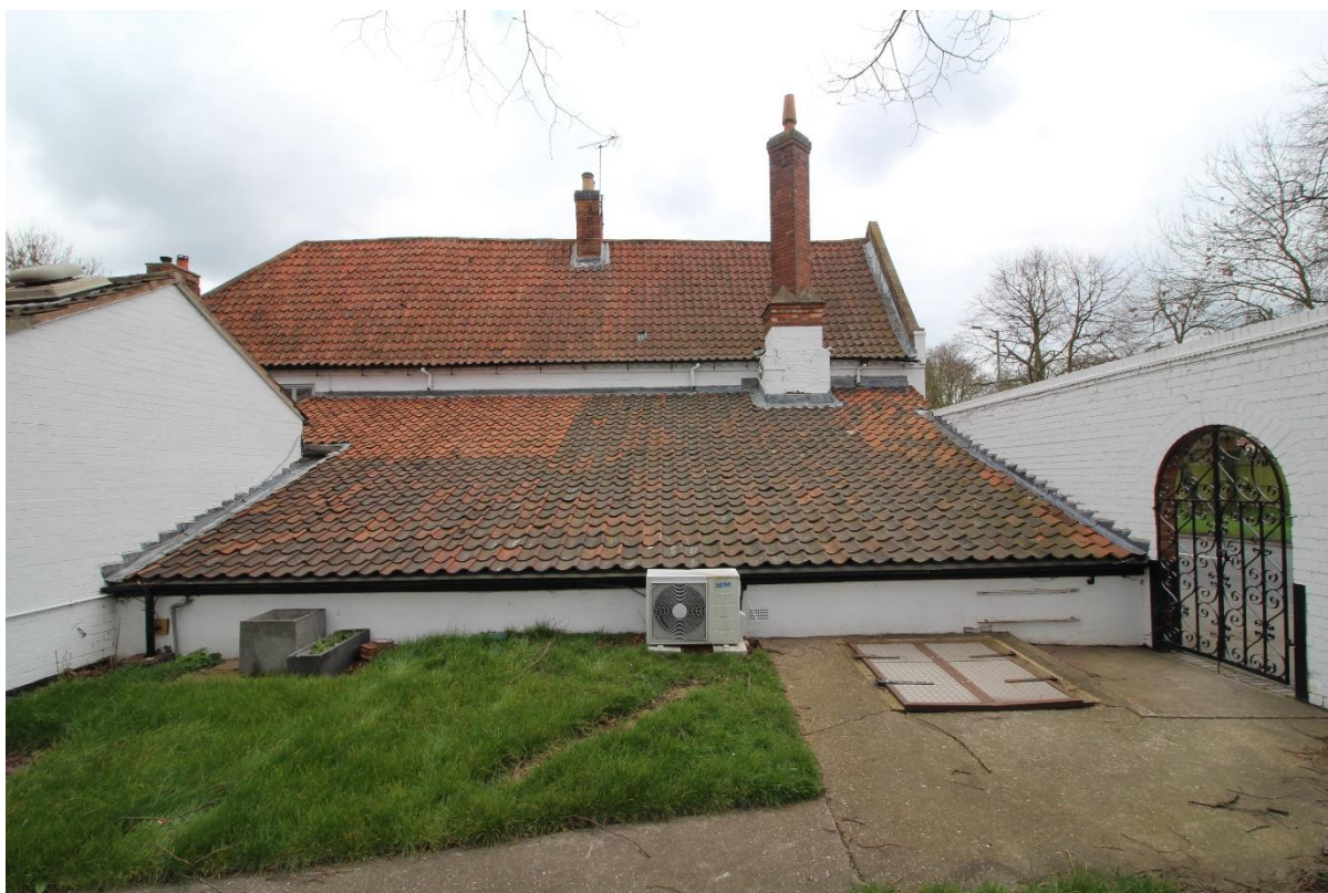
Figure 8 West elevation of the north-south range, looking east, note the outshot roof over the cellar
