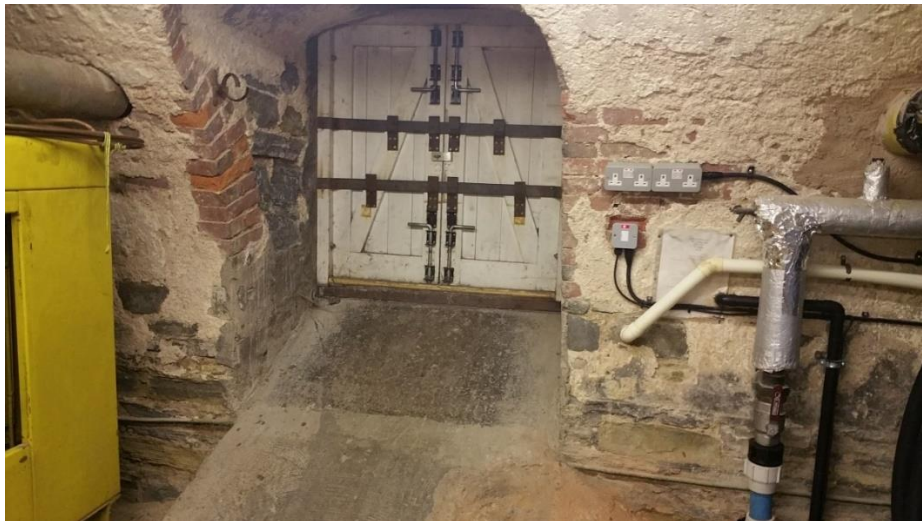
Complex mixture of construction materials in Area C – none of which matches that found in Area A or B (Location 22)
