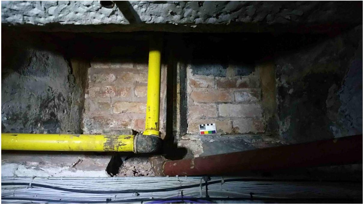
17th cent. Mullioned window high up on west wall of Area A – now bricked up and partially obscured by service pipes. (Location 7)
