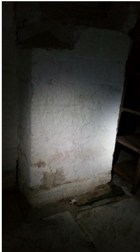
The Massive Central Pillar in Area A, viewed from W side – large finely dressed stones (3 ft. x 4.5ft footprint) – (Location 16)
