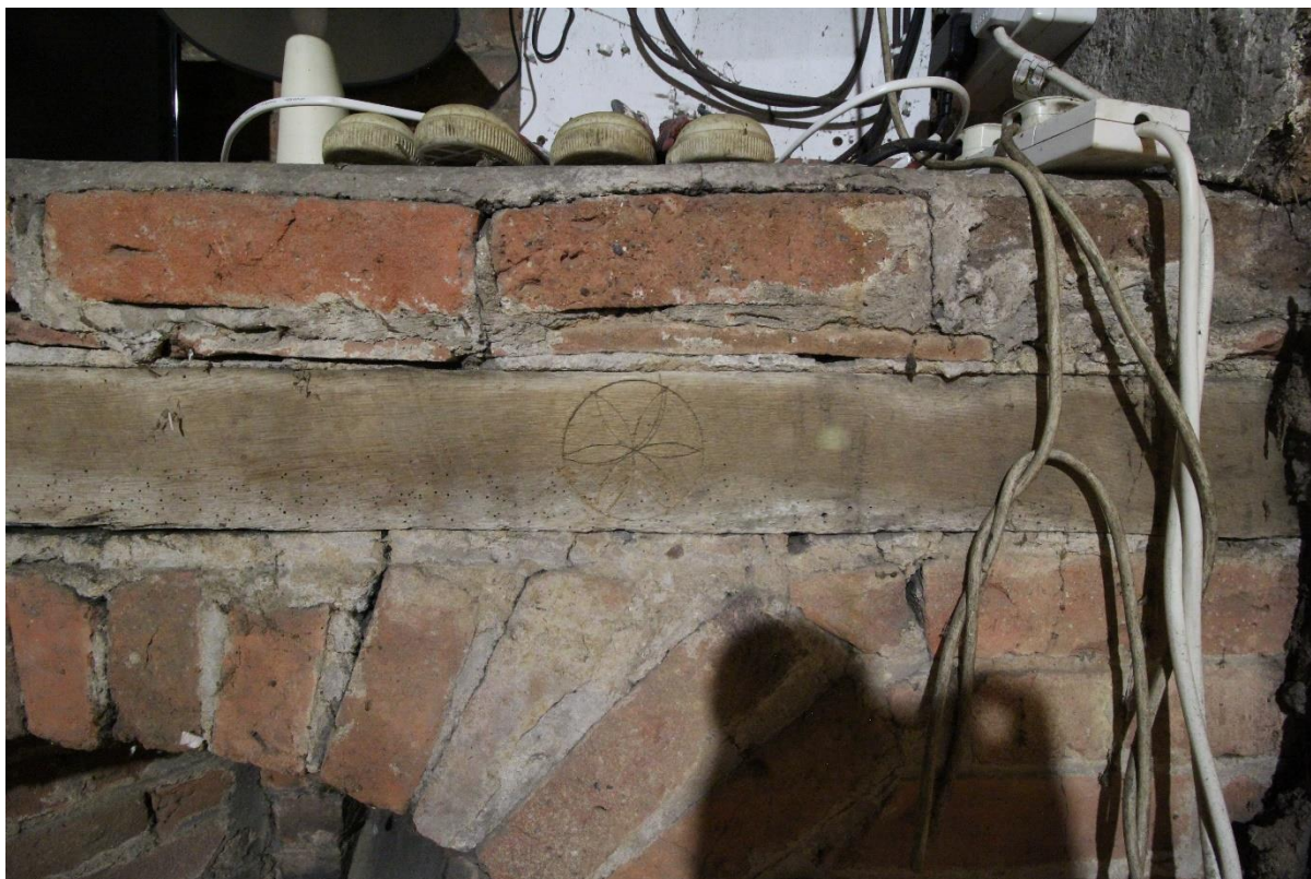
Figure 16 Daisywheel graffito on the timber lintel of the fireplace in the north elevation of the northern bay attic, looking north
