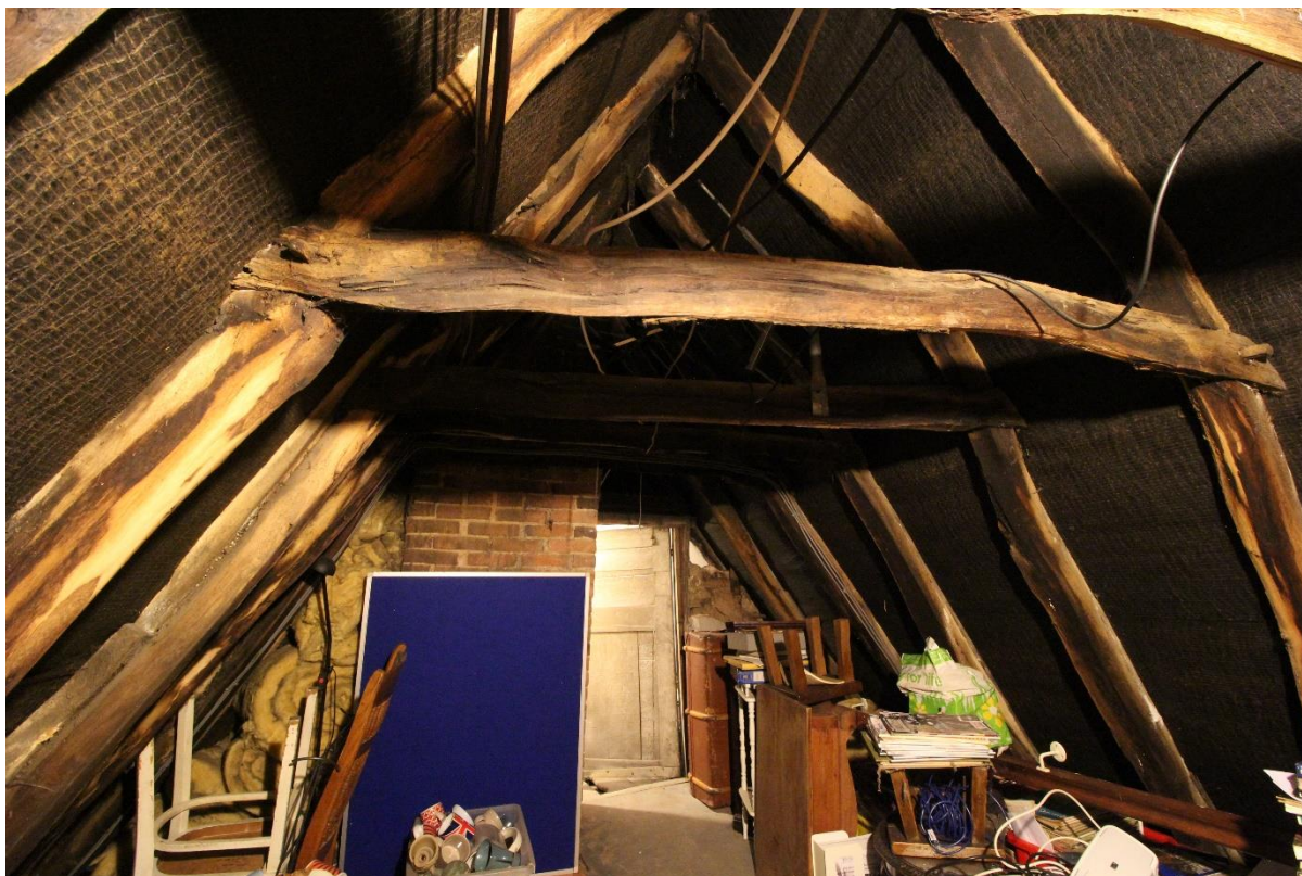
Figure 17 Roof structure of the central bay, note the smoke blackening of the timbers, looking south
