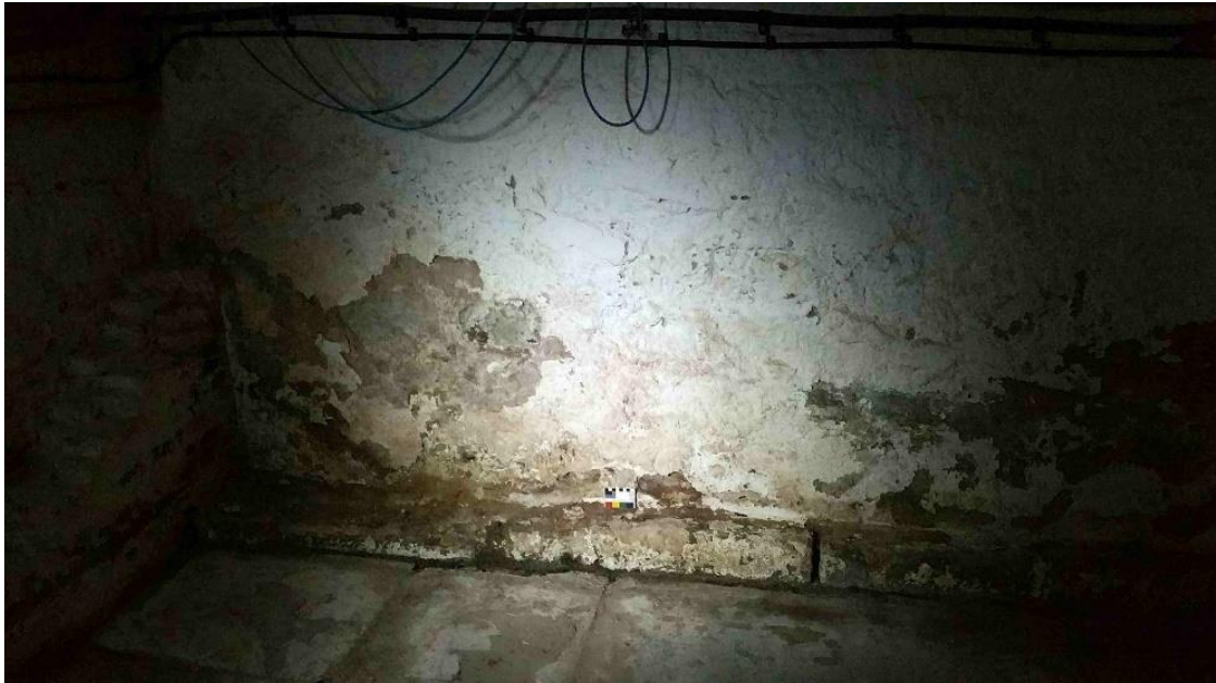
Misaligned foundation blocks below the N wall of B15 (Location 9)
